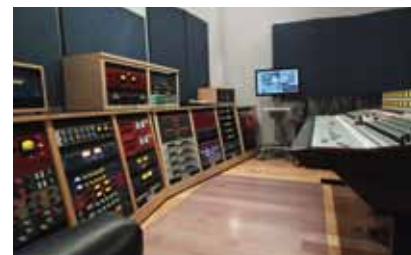
The Rupert Neve Designs 5088 analog mixing console installed at Mix One in San Francisco
